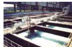
吸収廃液処理 Absorption liquid treatment system
